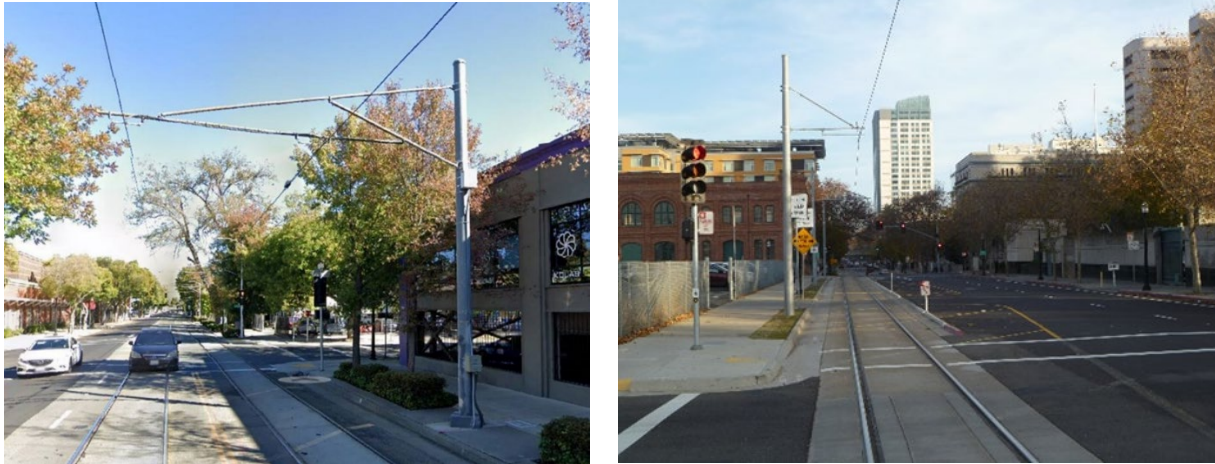
Figure 9 Photographs of Overhead Contact System
